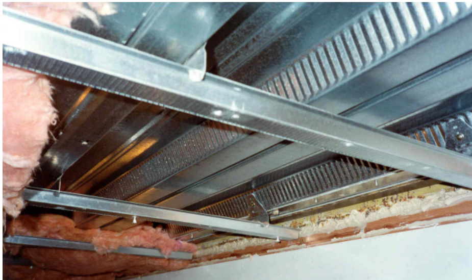
Figure 1: Underside of floor showing Hibond Steel Decking with USG direct fix clip and steel batten ceiling suspension system.
